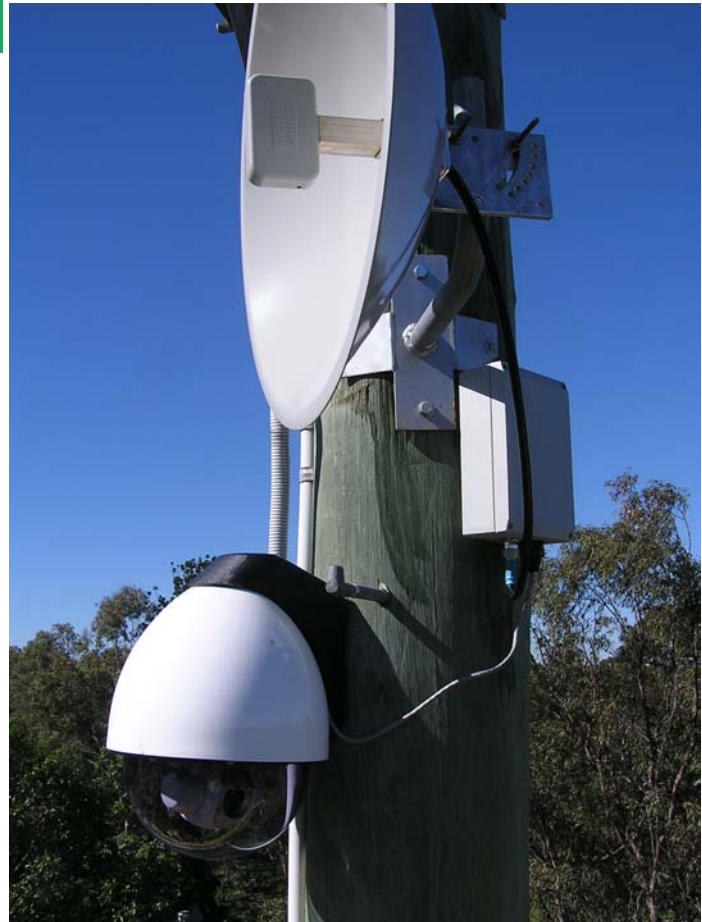
Shows installation of camera, with wireless and solar configuration on site.
